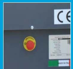
Emergency stop button it shuts down the generating set immediately
